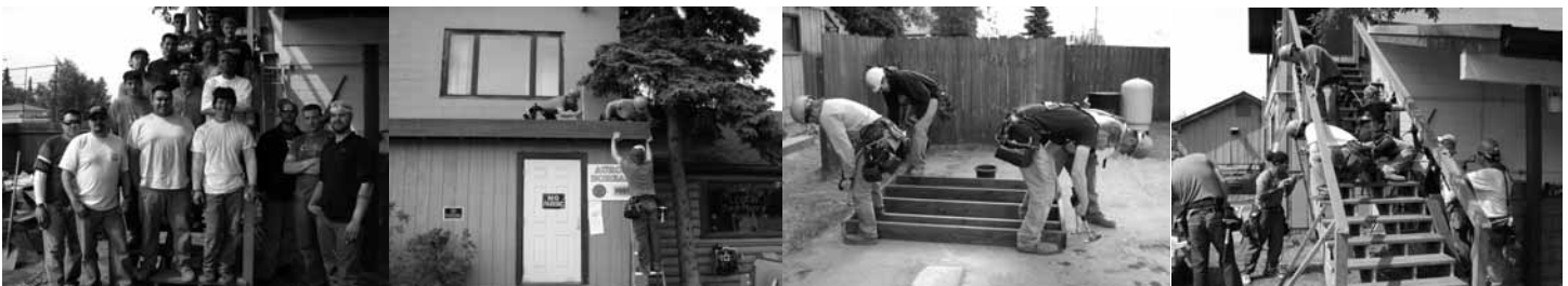
(Left) Brian Howe and Aaron Combs and all the first year apprentice volunteers that worked on the project. (Middle left) Philip Adajar, Sutin Le and Robert Wyckoff adding a new fascia board to the front entrance of the building. (Middle right) Sutin Le, Calvin Charlie, John Malaby, and Kevin Shields floor framing for deck on the back of the building. (Right) 1 st year apprentices putting on baluster for the stairs.
