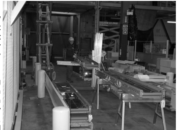
Apprentice Kendra Heidelberg preparing a conveyor for installation at USPS Bulk Mail Facility in Anchorage for Western Industrial Contractors
